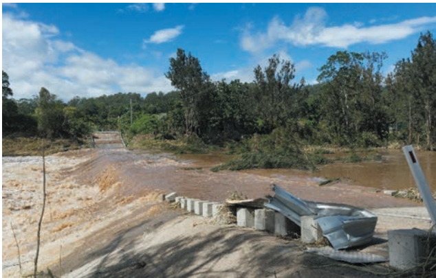
Figure 7. Flooded creek damaging roadway – Ex-TC Debbie, March 2017
