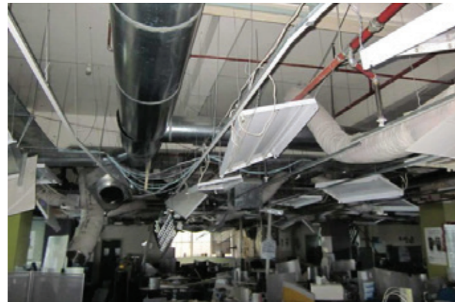
Figure 17: Widespread damage resulting from a ceiling failure after a Canterbury earthquake. Source: Geoscience Australia
