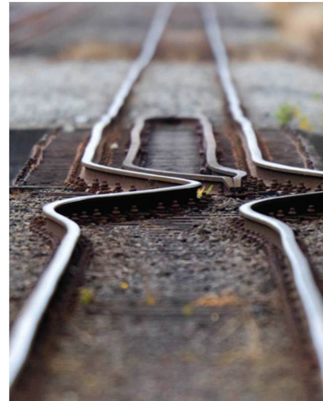
Figure 11: A rail line buckled by the shifting earth is pictured in Christchurch on February 23, 2011. Source: Getty Images
