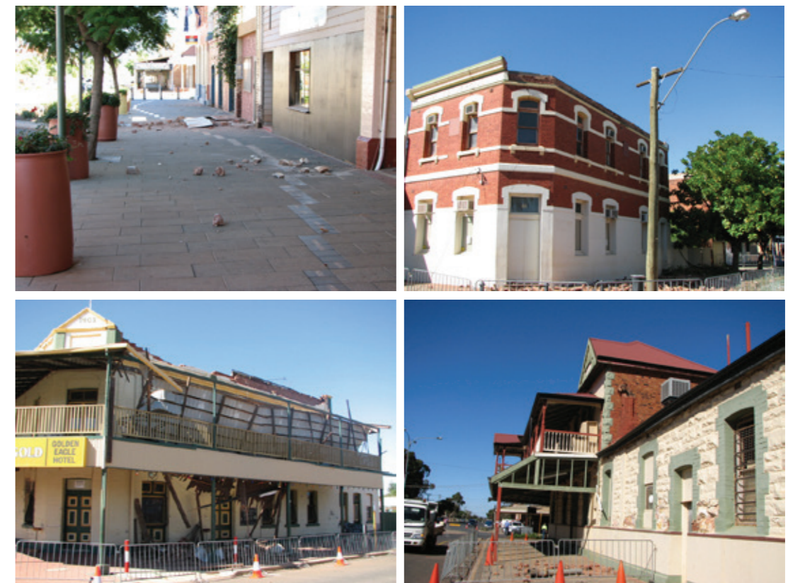
Figure 14: Damage sustained within the town of Kalgoorlie-Boulder, Western Australia as a result of the magnitude 5.0 earthquake which occurred on 20 April 2010. Source: images courtesy of Department of Fire and Emergency Services, Western Australia
