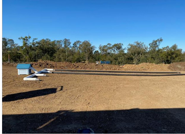
HEAPS setup showing pipes and fan
