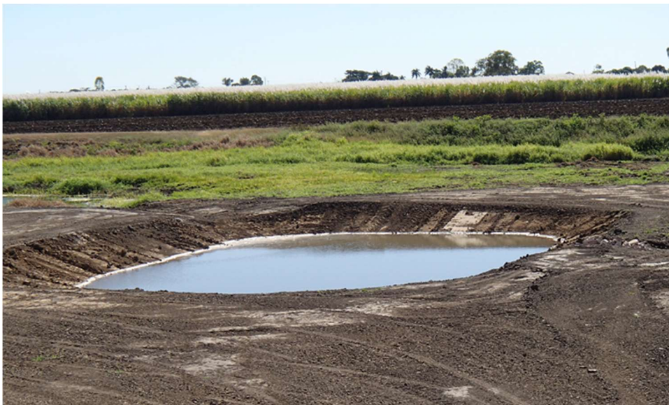
Figure 7: Top: Diagram to show how a sediment basin captures run-off water. Bottom: A newly constructed sediment basin (Source WetlandInfo 2018c).
