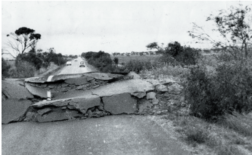
Figure 2: Road buckled by the shifting earth from the Meckering earthquake 1968. Source: West Australian Newspapers Limited
