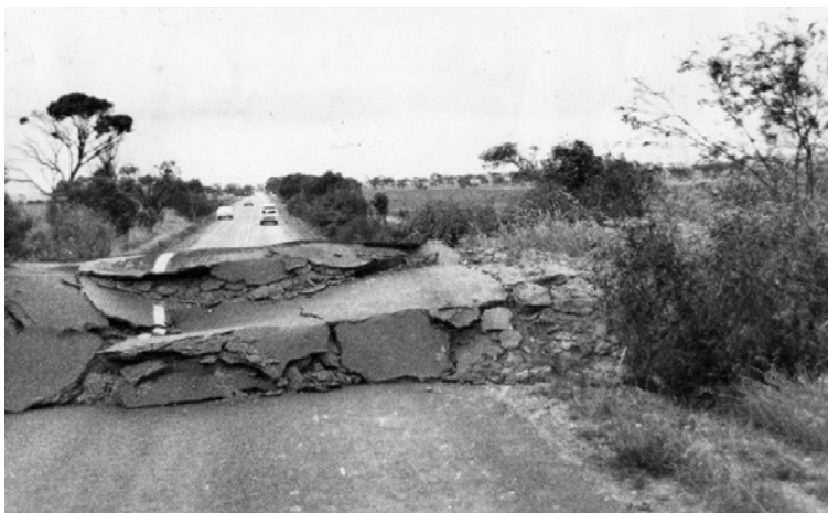
Figure 13: Road buckled by the shifting earth from the Meckering earthquake 1968. Source: West Australian Newspapers Limited.
