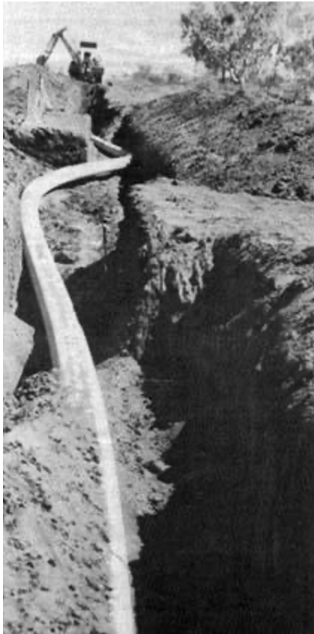
Figure 11: Gas pipeline warped by ground rupture from the Tennant Creek Earthquake in the Northern Territory 1988.
