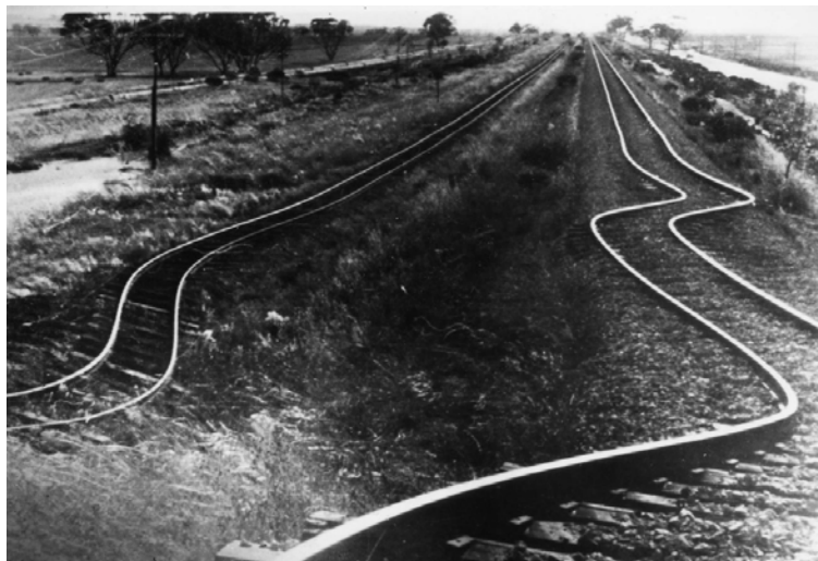
Figure 12: Rail line buckled by the shifting earth from the Meckering earthquake 1968. 1968 Meckering – Australian Earthquake Engineering Society (aees.org.au)
