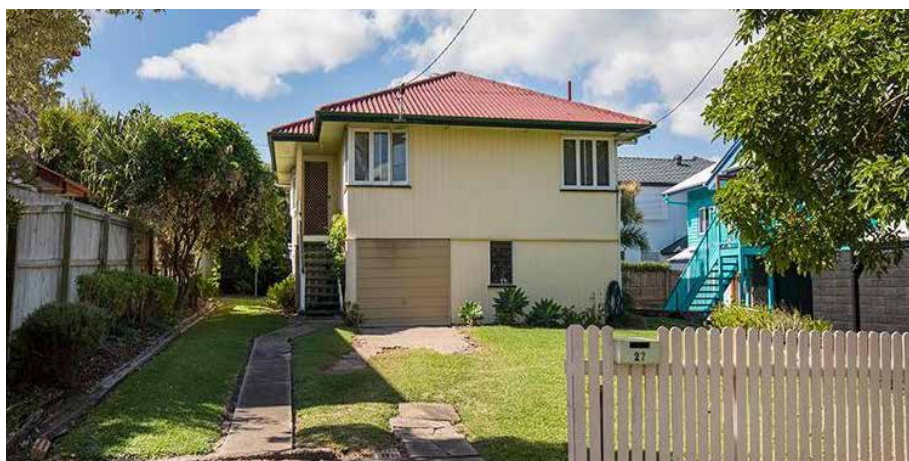
Figure 15A: An example of a post-war house. Its timber frame makes it quite resilient to earthquake shaking, however the fibrolite roof could become a significant environmental hazard if it were damaged in an earthquake. Source: Adobe images
