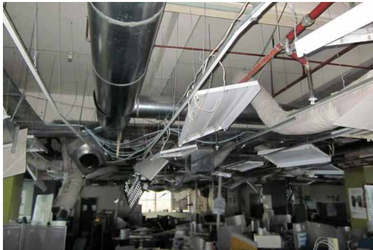
Figure 16: Widespread damage resulting from a ceiling failure after a Canterbury earthquake. Source: Geoscience Australia
