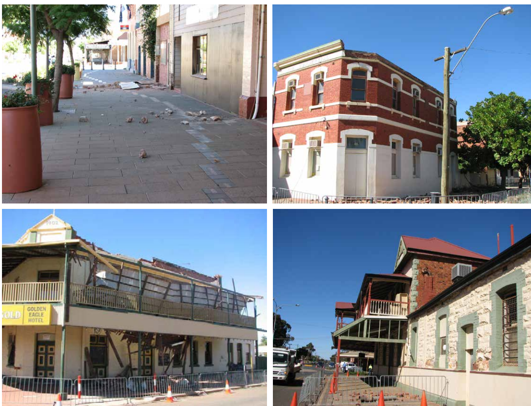
Figure 14: Damage sustained in the town of Kalgoorlie-Boulder, Western Australia as a result of the magnitude 5 earthquake (20 April 2010). Source: Department of Fire and Emergency Services, Western Australia
