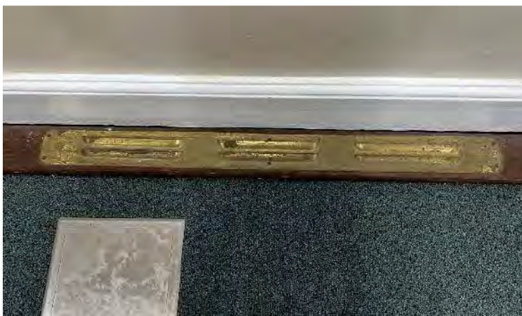
Figure 72: Brass vents alongside the skirting board (AHS 2021).
