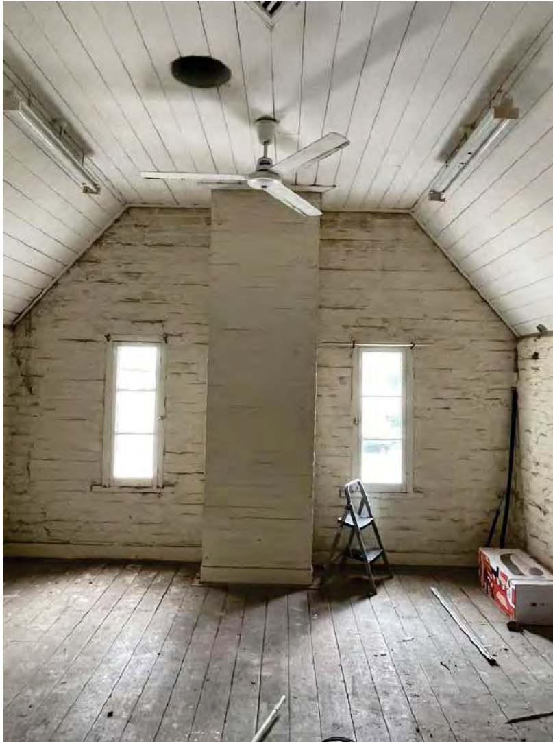
Figure 113: Room 16 facing west showing brick chimney and walls, timber floorboards, VJ ceiling, and casement windows (AHS 2021).
