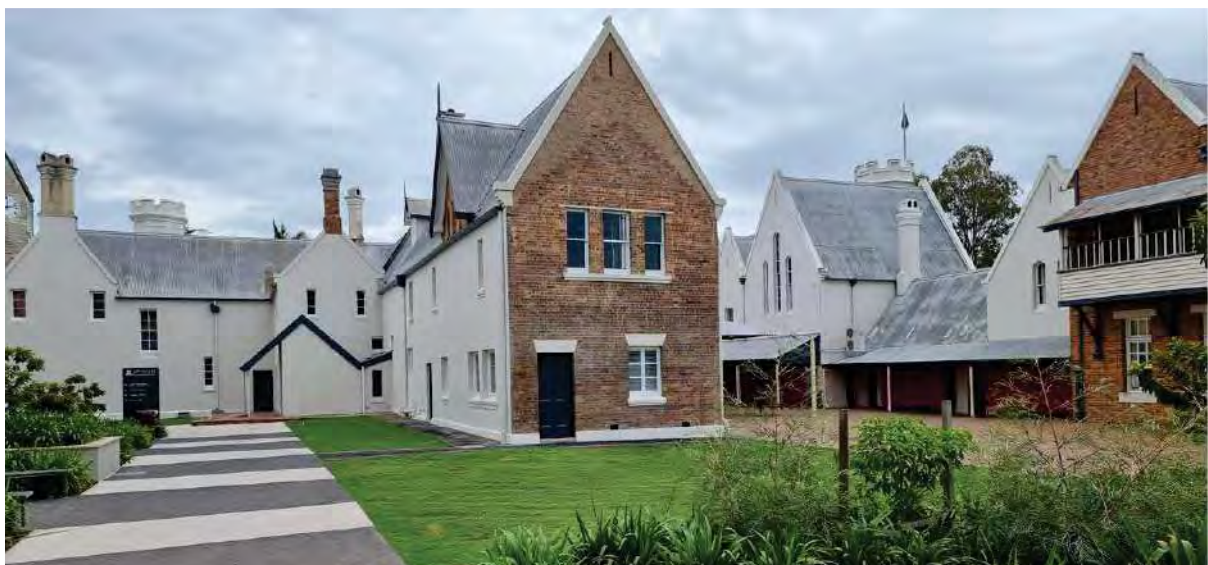
Figure 51: Western elevation showing 1877 extension and courtyard (right) showing the repair and re-render of the northern elevation of the 1877-extension (IGS, 2021).
