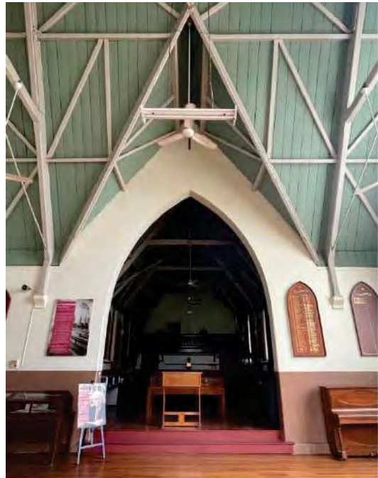
Figure 59: Great Hall facing north showing the intersection of the 1863 portion (1b) and 1865 portion (1a) to create a T-shape. Photograph was taken in section 1a (AHS 2021).
