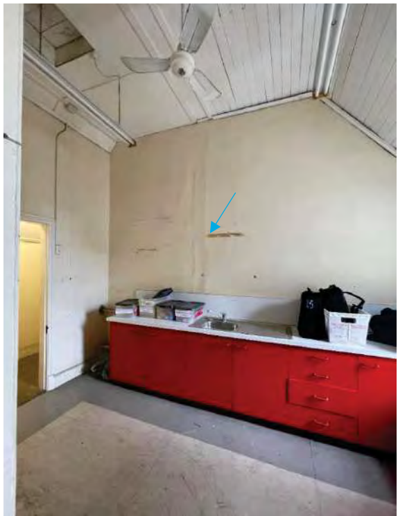
Figure 109: Room 15 showing red kitchenette, vinyl flooring, and dual ceiling. The former wall is indicated with a Blue arrow (AHS 2021).
