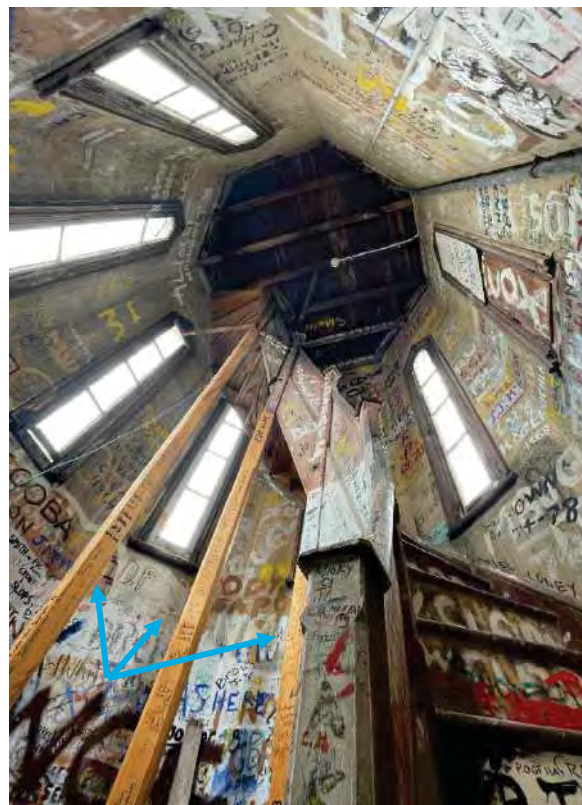
Figure 95: Upper tower winding staircase. Note the replaced support posts to the staircase [Blue arrows] (AHS 2021).
