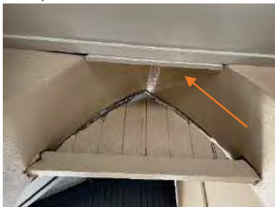
Figure 67: Decorative VJ panels in archway leading to courtyard. Note the new ceiling cuts into the arch [Orange arrow] (AHS 2021).
