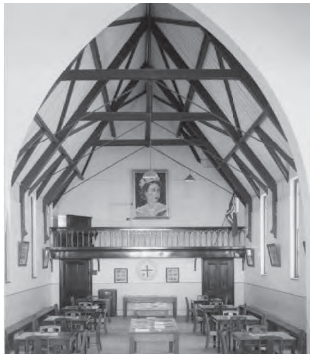
Figure 164: Great Hall, 1954 (Ipswich Library, Reference No.: WHD-014-NEG-0965p). Note that the hall has a lighter colour scheme, with the dado rail delineating the lower wall colour. The timber roof structure has also been painted a darker colour. The piano has been moved to the gallery space, and a large portrait of Queen Elizabeth II is mounted in the centre, likely due to the 1954 Royal Tour.
