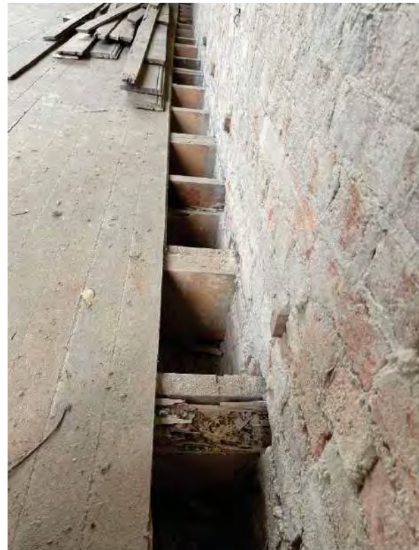
Figure 100: Floorboards removed to reveal termite affected timber bearers (AHS 2021).
