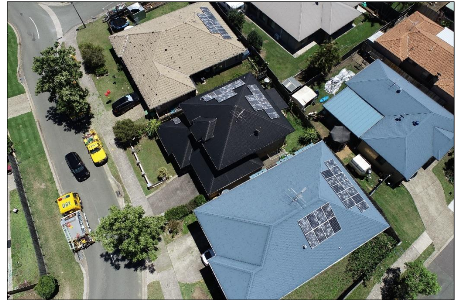
Figure 13: Drone footage of damaged solar panels and roofs in Ipswich. The damage was caused by severe weather experienced in South East Qld on 31 Oct 2020. Image: QFES.
