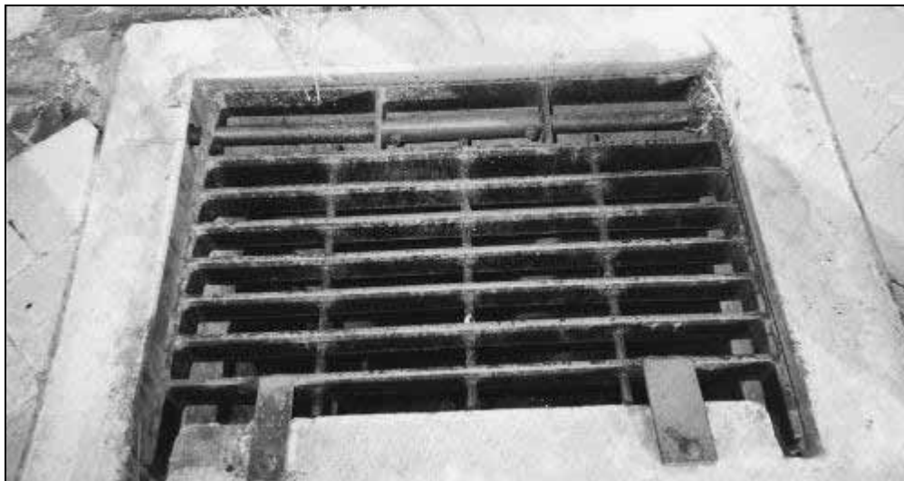
Photograph 7.23: John Oxley Youth Detention Centre stormwater grate where a boy was handcuffed overnight—Inquiry photograph
