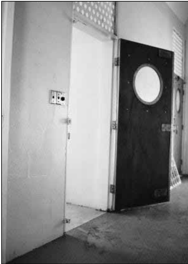
Photograph 7.20: Cell door with steel mesh (potential hanging point) (1999)—Inquiry photograph
