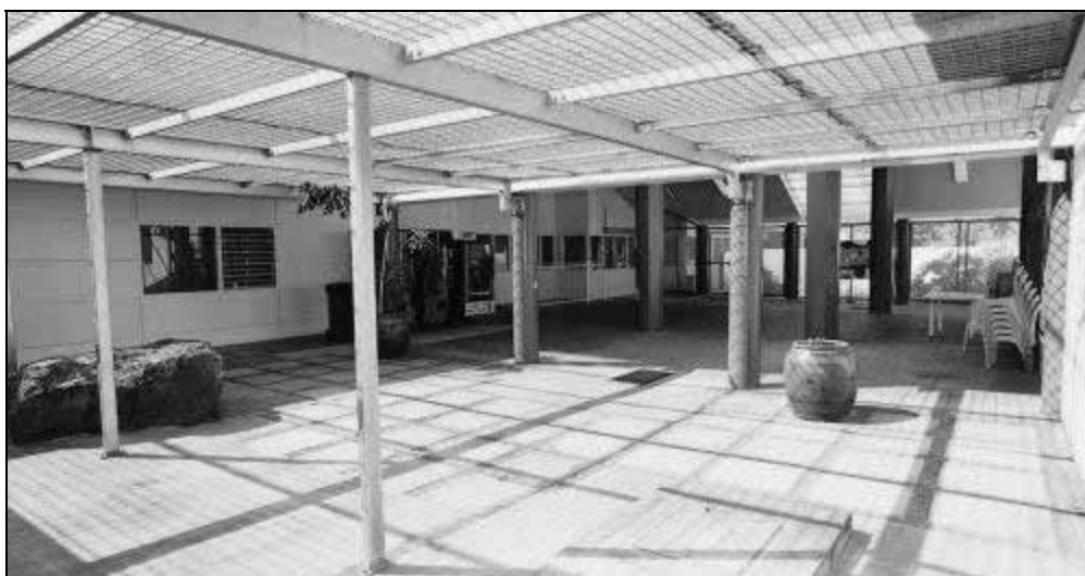
Photograph 9.12: John Oxley Youth Detention Centre visiting area is spacious and provides a food/drinks machine, but still feels like a cage—Inquiry photograph
