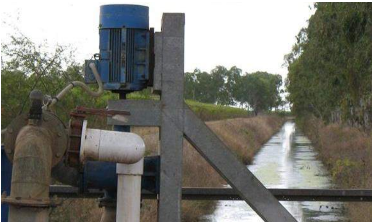
Figure 86. Pumping from a recycle pit – lower Burdekin
