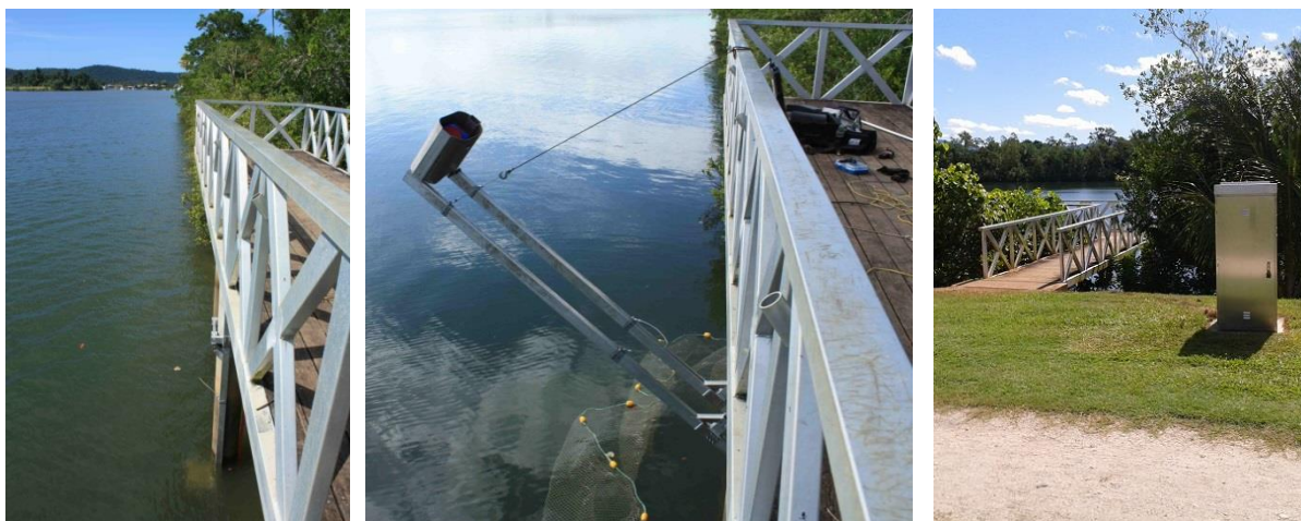
Figure 2 The H-ADCP swing arm locked in the monitoring position (left), the H-ADCP being raised on the swing arm for maintenance (centre) and the flow site's secure housing (right)
