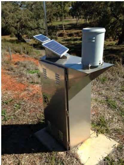
Figure 3.6 TYPICAL RAIN AND WATER LEVEL STATION WITH SOLAR PANELS
