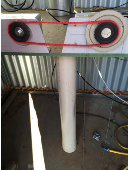
Figure 3.3 WET WELL SHAFT ENCODER
