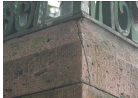
The rusting iron arch embedded in this gate pillar has expanded, causing the capital to crack.
