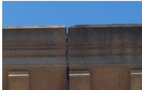
Mortar lost from the joints between the uppermost blocks of this memorial will allow water to enter the memorial instead of falling clear of the side. This may eventually damage the stone.
