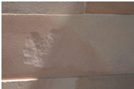
The markings on this damaged stone suggest it has been cleaned with an abrasive power tool.
