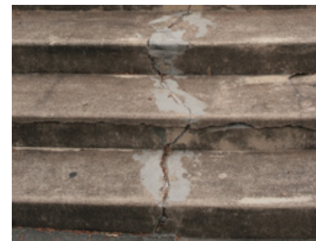
The crack in these concrete steps has probably been caused by ground movement or root growth from nearby vegetation.
