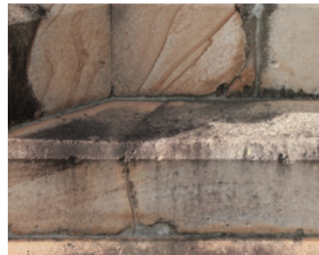
This crack has travelled across sandstone blocks and may be the result of ground movement. Water has penetrated the crack and contributed to crumbling of the stone. Mortar has been used to patch damaged stone towards the bottom of the picture.
