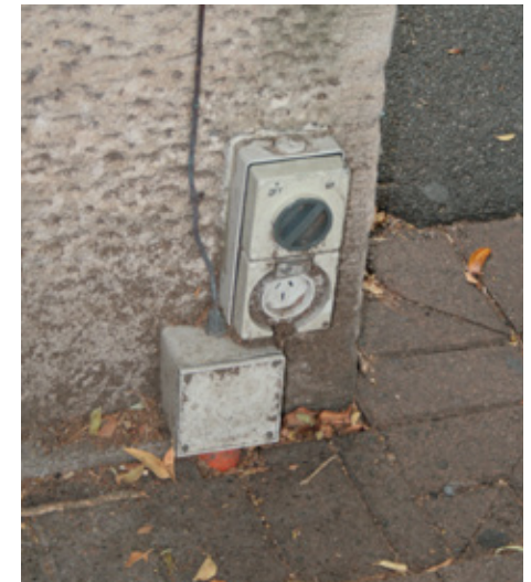
Do not fix services such as electrical outlets to stonework.
