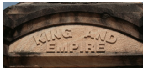
Sandblasting this memorial resulted in loss of definition of the lettering (top). The section of stone bearing the lettering was later replaced (bottom).
