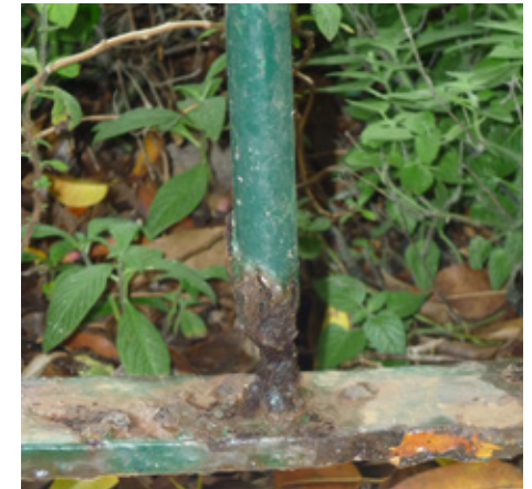
This iron picket has almost rusted through. It will be necessary to treat the rust and replace the lost metal with metal replacement filler or to remove the badly corroded section and weld a replacement section.
