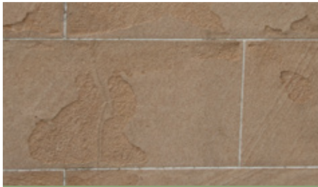
The face of this stone is delaminating.
