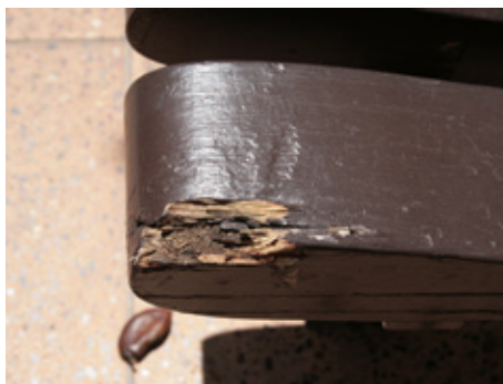
Fungal wood rot in the armrest of a timber seat at a memorial.
