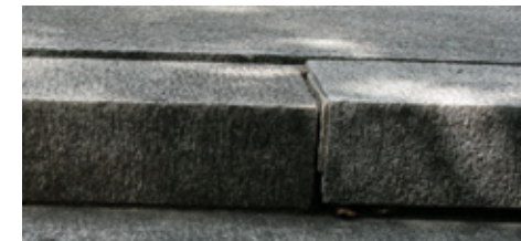
These granite slabs have been disrupted by the roots of trees growing nearby.
