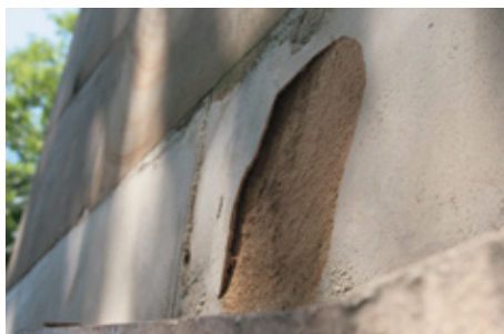
The long-term effects of applying an anti-graffiti coating to sandstone: the outer layer of stone has lifted.
