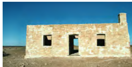
For example, the stone ruins of Carcory Homestead (c1877) in the Diamantina, have the potential to reveal important information about stone construction in the Australian interior in the second half of the 19th century.
