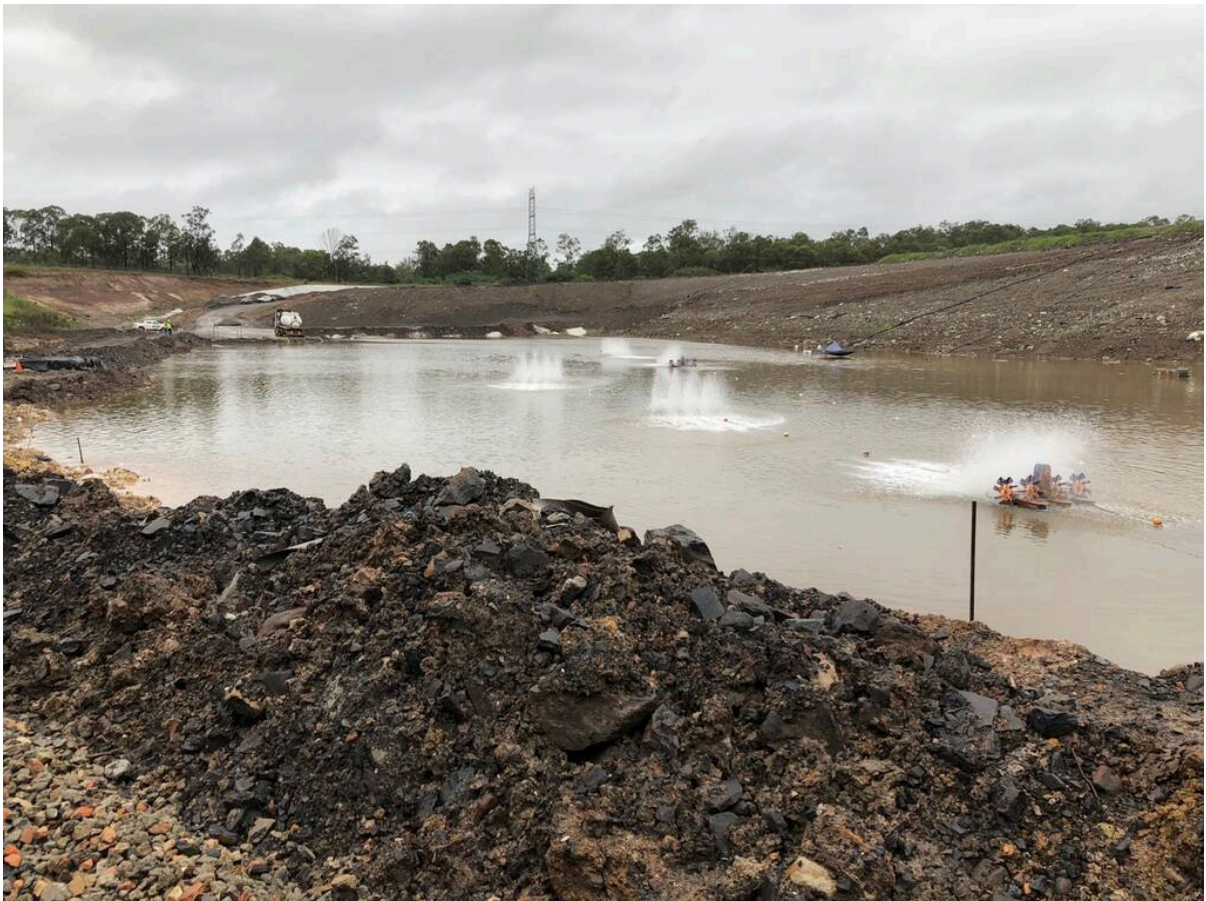
Looking at the affected cell from the northern end in May, when the water level was about 26ML. This was prior to the second rain event.
