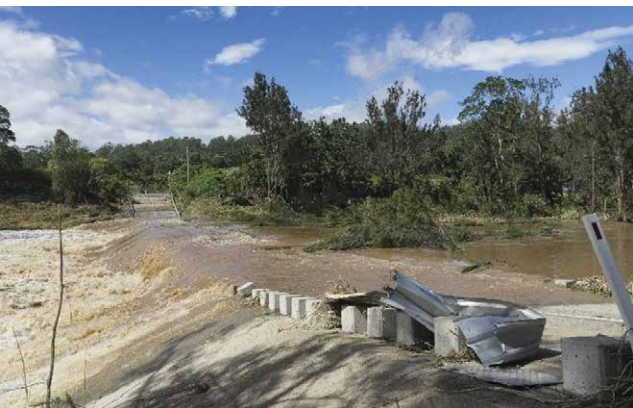
Figure 17. Flooded creek damaging roadway – Ex-TC Debbie, March 2017
