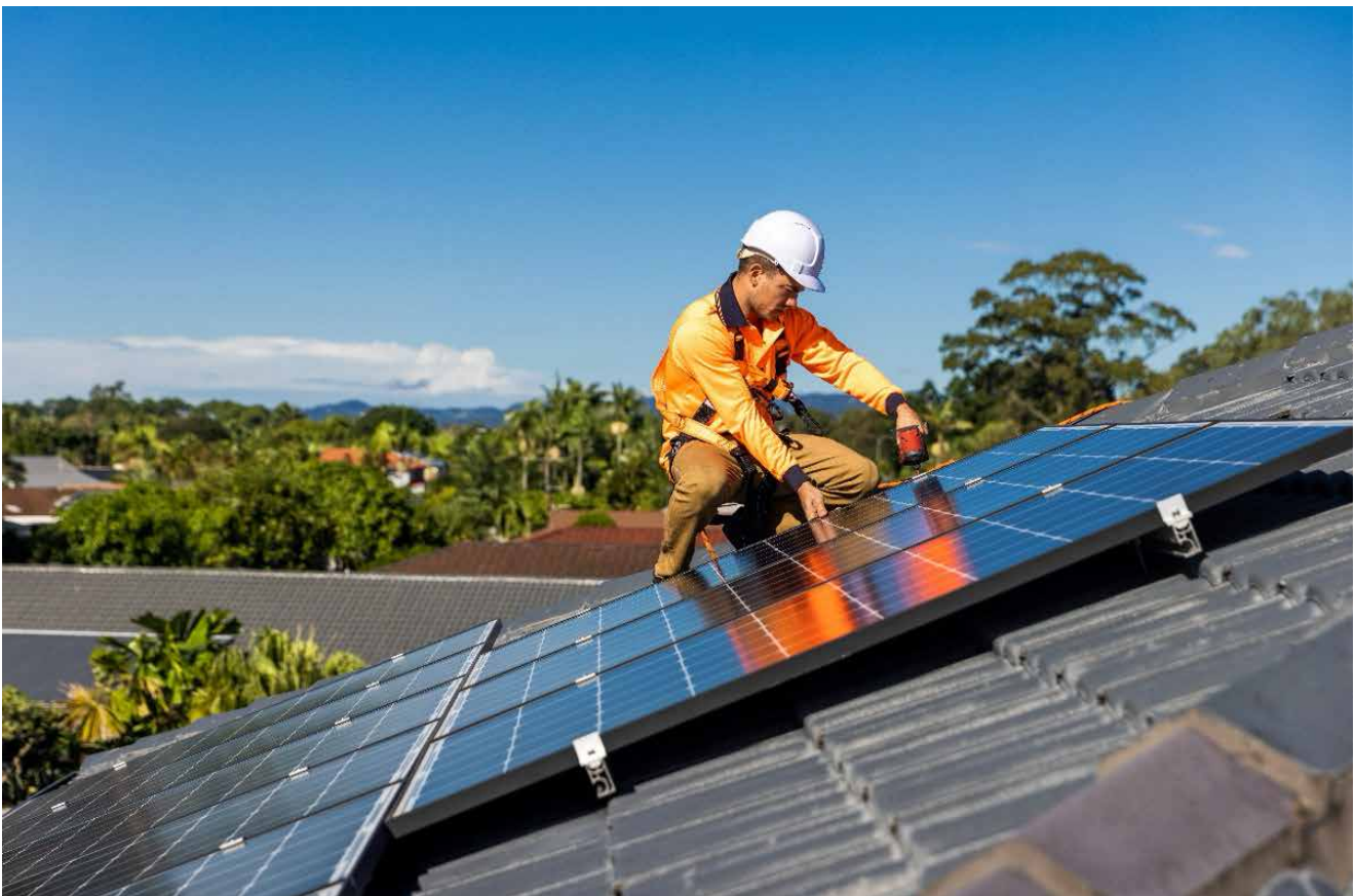
Figure 11. Solar power installation is increasing across Queensland.
